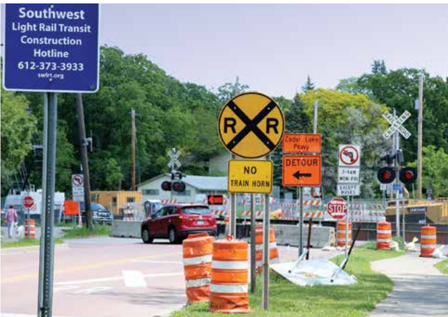
SWLRT Detour as work progresses at Cedar Lake Parkway and the Kenilworth Trail 2022
