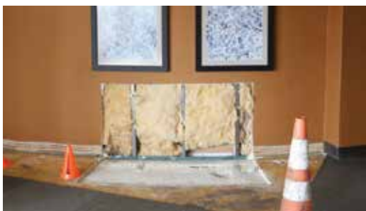
Cracks throughout building with exposed walls and floors for monitoring. (Photo Dorothy Childers.)
