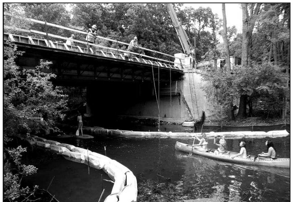
Workers chatted with canoeists and paddle-boarders on the Kenilworth Channel while waiting for the next cement truck to arrive. Channel closures during construction have been minimal, and workers hope they can remove the wood framework supporting the rebar without closing the channel.
