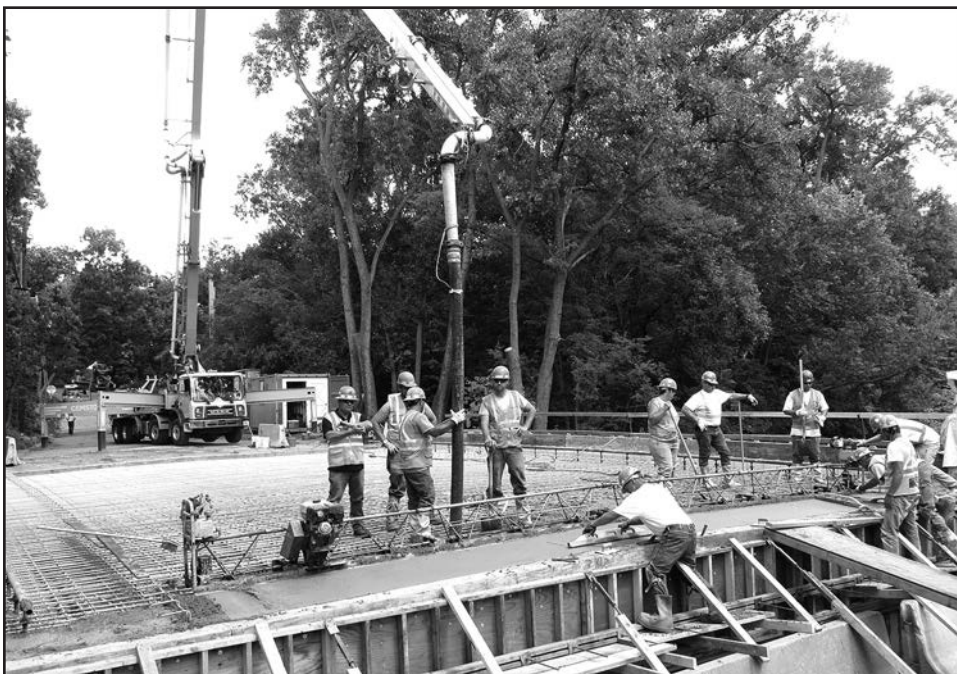
Workers took advantage of perfect summer weather on July 21 to begin pouring 112 cubic yards of concrete onto the prestressed concrete beams and rebar of the deck of the new Burnham Road bridge. The concrete will require about seven days to cure. Kraemer NA hopes to complete the bridge by mid-August so that city crews can begin to rebuild short stretches of the roadway on both sides of the bridge. If all goes as planned, Public Works officials say the bridge could reopen October 1.
