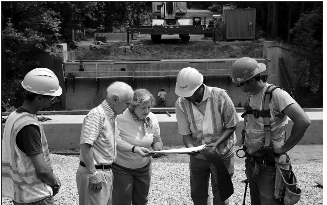
Hassan Nur (second from right), Department of Public Works engineering technician, met with Park Lane residents Fred and Gloria Sewell for an update on the Burnham Bridge replacement while Dale Murphy (left), Kraemer North America labor foreman, and DPW intern Bassam al-Mohamadi, a senior Civil Engineering student at MN State University/Mankato, listened in. Pleased with the bridge replacement, the Sewells said, "This is progress. This is good." (Photo: Dorothy Childers. Caption: Michael Wilson)
