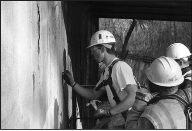
City workers take concrete soundings under the Burnham bridge in May, 2014, to determine extent of deterioration.
