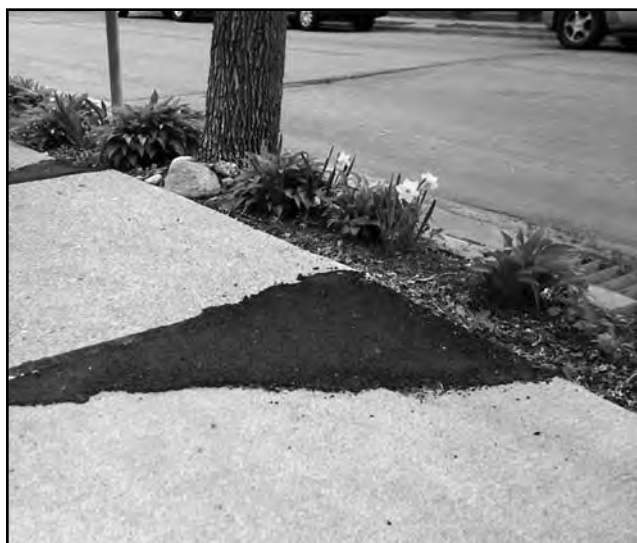
Temporary asphalt patches on Douglas Avenue in Lowry Hill
